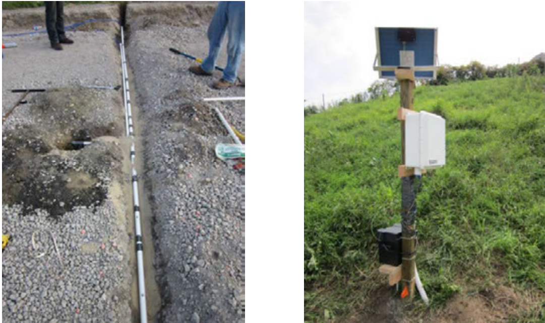
Figure 54. U.S. Highway 30 vertical and horizontal temperature probes (left) and temperature probe data acquisition set up (right)
